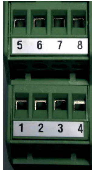
connections for PLC/Power Circuit
