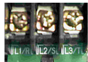
connection of main circuit power input terminals (from contactor with protection switch)
